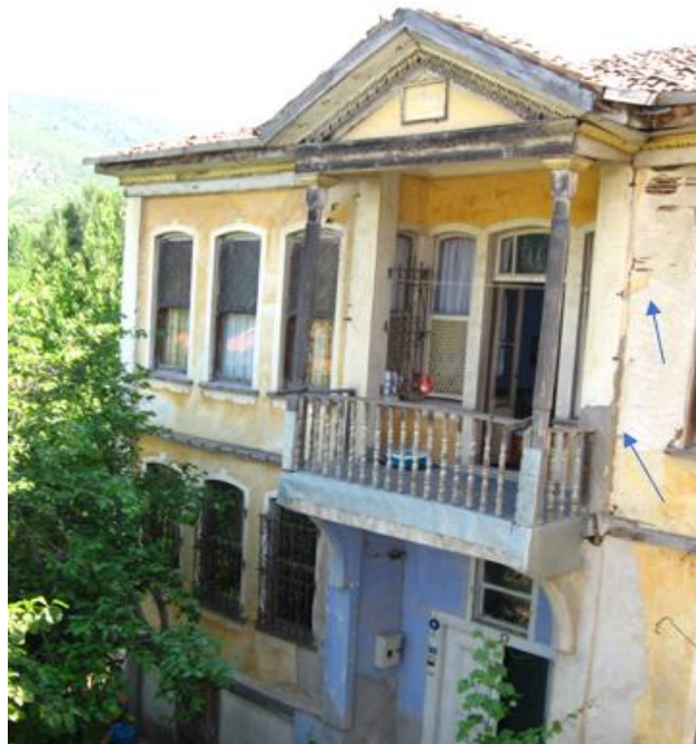
Figure 5. Ayşe Sezgin House of Deteriorations caused by the effect of heat on the exterior of the structure.
