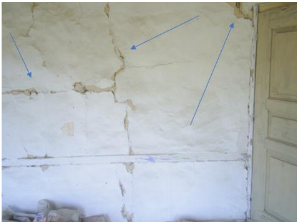
Figure 15. İbrahim Pilavcı House of crack caused by mechanical action on the wall surface.
