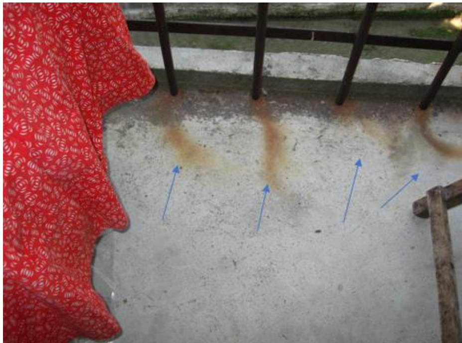
Figure 13. Ayşe Sezgin House of corrosion induced deterioration in flooring.
