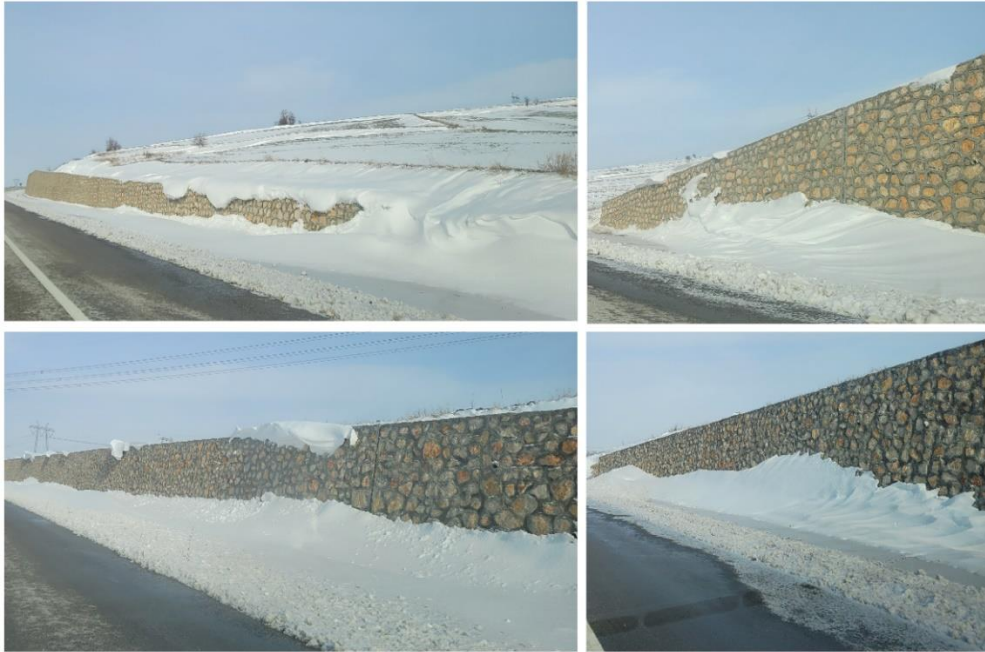
Fig. 6. Photographs of snowdrifts on the water channel and anti-erosion walls due to snowfall and snow plowing from the road on February 6-7, 2023.
