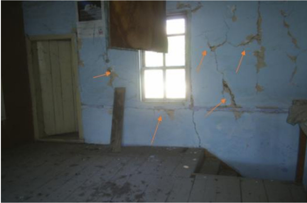
Figure 16. İbrahim Pilavcı House of crack caused by mechanical action on the wall surface.
