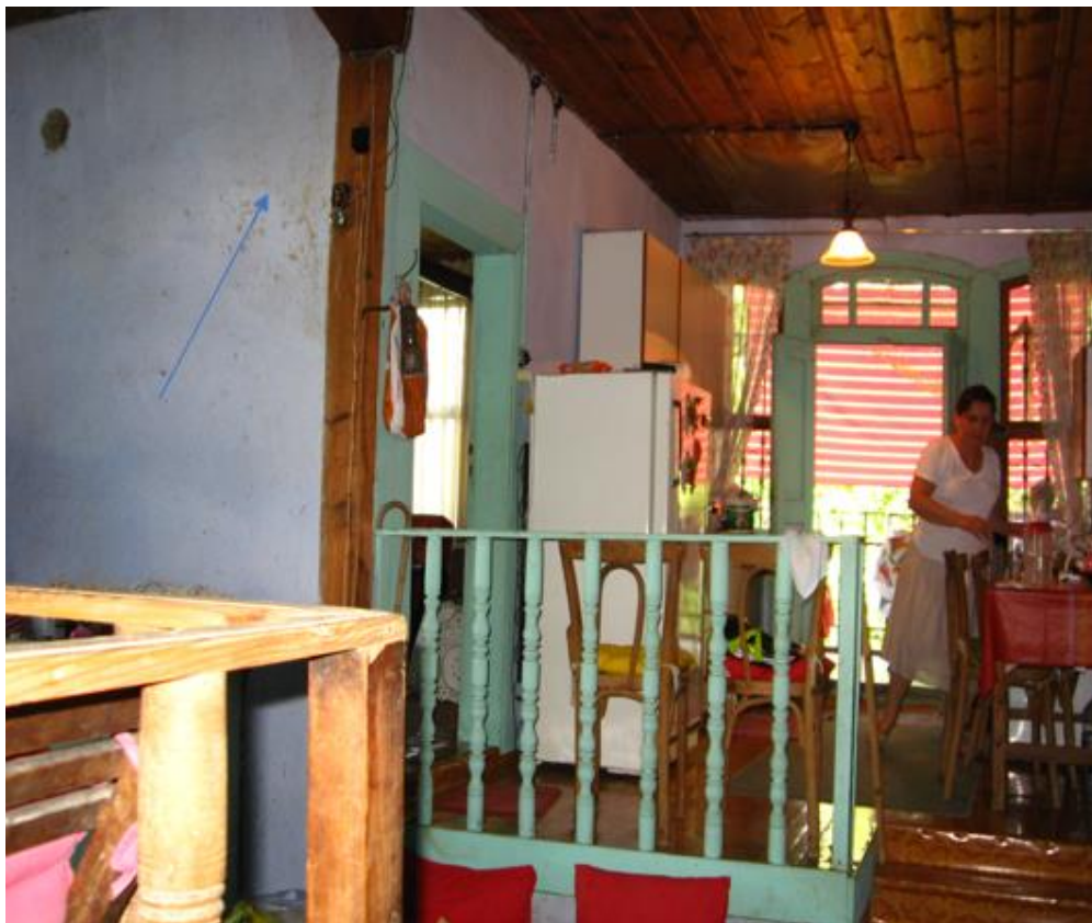
Figure 11. Ayşe Sezgin House of deterioration of the wall surface due to water and moisture.
