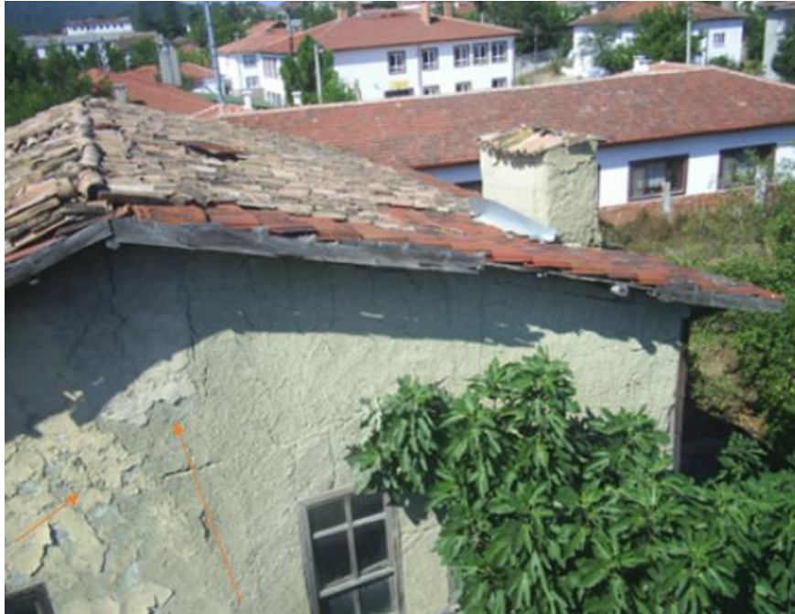
Figure 6. İbrahim Pilavcı House of deteriorations caused by the effect of heat on the exterior of the sturcture.
